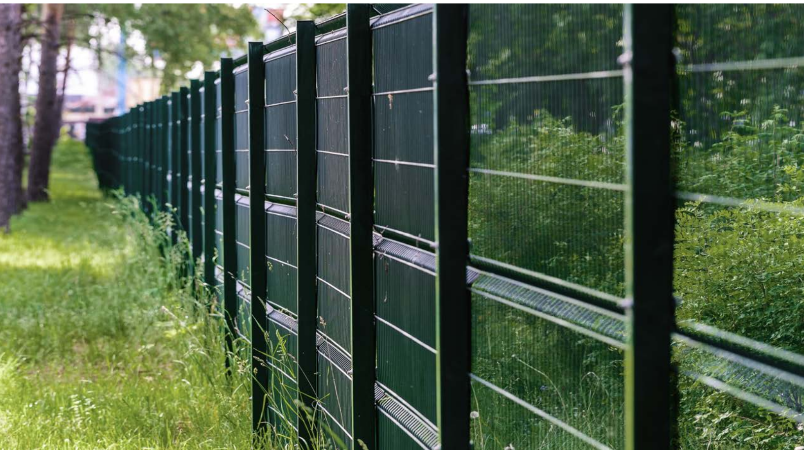
High Security Welded Wire Mesh Fence
